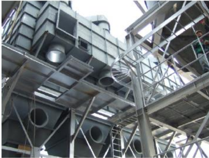
<Filtration Interior facility after coating>
